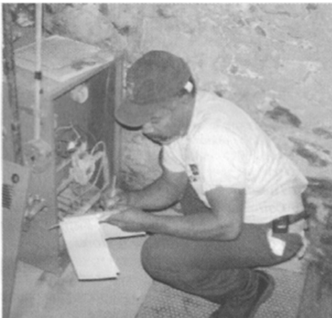
A repair man tends to a damaged furnace. Dialing down your thermostat, especially at night, is one of several ways to reduce energy costs.
