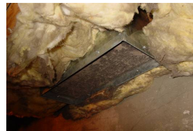
Figure 3113-2: Dirty combustion air intake to wood stove that needs to be cleaned
