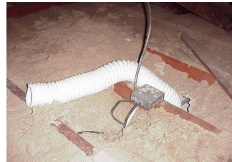
Figure 507-1: Fans may not be vented into the attic under the Weatherization Program
