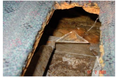
Figure 4114-1: Opening between duct boot and floor
