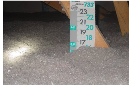
Figure 2138-1: Attic insulation marker
