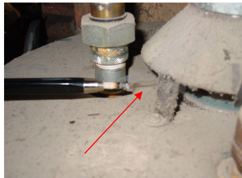
Figure 117-1: Conducting a spillage test with a smoke pencil – passes
