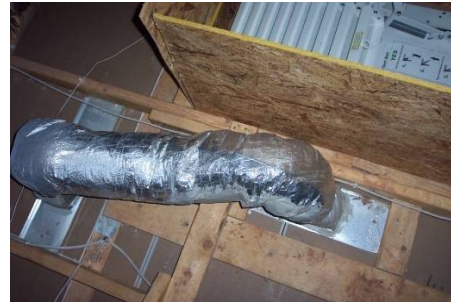
Figure 1153-1: Jumper duct installed in attic connecting bedroom to hallway (Courtesy Southface Institute)
