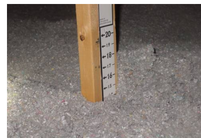
Figure 21331-2: Attic insulation marker
