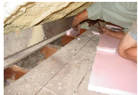
Figure 21364-4: Connecting roof thermal boundary to sidewall thermal boundary with rigid foam board insulation; 2-part spray foam will also work
