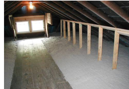
Figure 21332-1: Insulation blown under floor boards and then over floor boards where client storage is not needed
