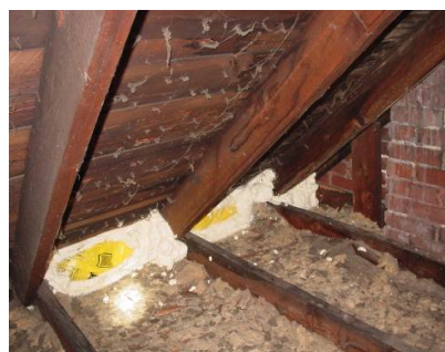
Figure 2122-5: Balloon framed stud cavity sealed with fiberglass batts stuffed in cellulose insulation bags
