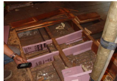
Figure 2131-5: Rigid foam board used as barrier next to K&T wiring; floor cavity will be blown with cellulose insulation
