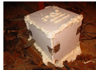
Figure 2131-1: Recessed light covered with drywall box
