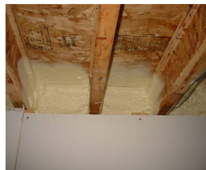
Figure 2171-1: 2-part spray foam on rim joist
