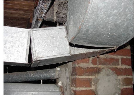
Figure 31531-3: Seal leaks and connections in supply and return ducts
