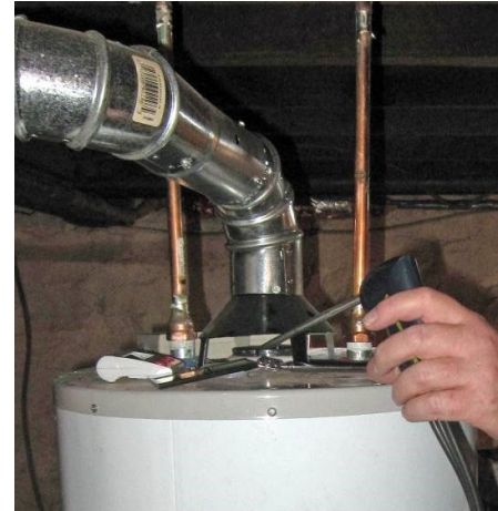
Figure 3123-1: CO reading taken for water before dilution air
