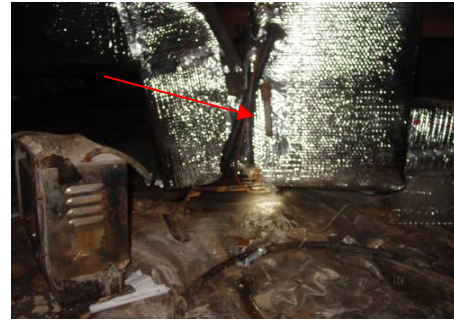
Figure 2154-3: Condensate line draining on top of ground moisture barrier
