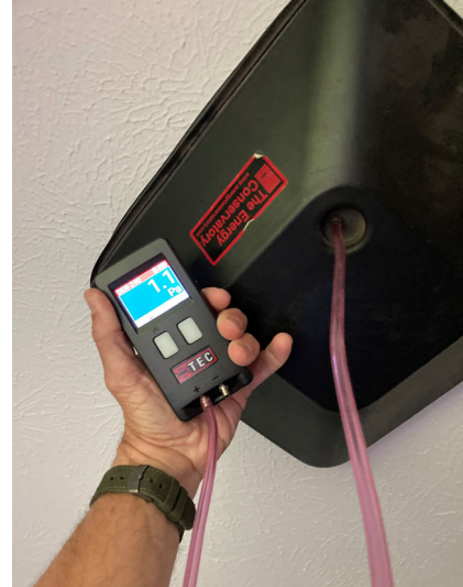
Figure 1142-1: Tight duct measuring 1.1 Pa
