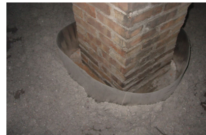
Figure 2131-3: Metal barrier around chimney
