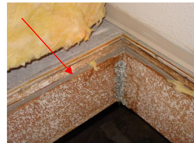
Figure 2153-1: Peel & stick weatherstripping is not permitted
