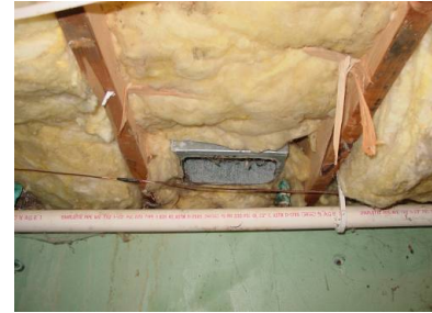
Figure 2151-3: Combustion air intake from crawl space; floor above crawl space is thermal boundary
