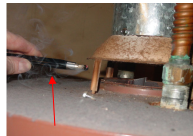
Figure 3122-2: Appliance fails spillage test
