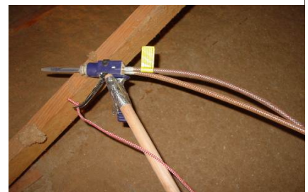
Figure 2122-12: 2-part spray foam gun secured to broom stick with string attached to handle
