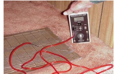
Figure 41144-1: Initial pressure pan reading of 47 Pa; return duct was totally disconnected
