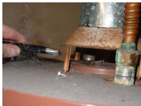
Figure 117-2: Failed spillage test
