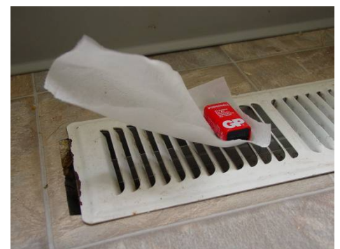
Figure 1141-3: Sometimes duct leakage is obvious before you use the pressure pan; air coming out of a register with blower door operating; air handler is not on!
