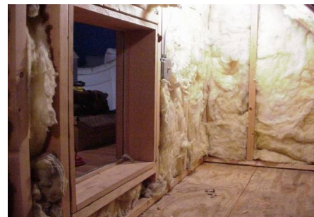
Figure 21364-1: Knee walls insulated with fiberglass insulation
