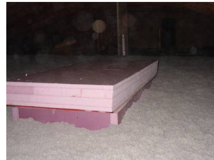
Figure 2135-1: Attic hatch insulated with foam board; plywood blocking has been insulated with foam board
