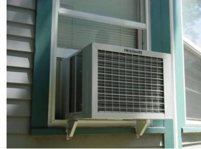
Figure 3156-1: Room air conditioner
